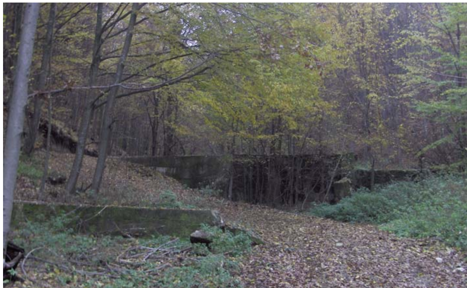
Fig. 6. 7 Lucrarea 3B0/2,0, aval de lucrarea 4B3,0 de pe Valea Rea (foto: Tudose 2009). Works no. 3B0/2.0 located downstream no 4B3.0 on Valea Rea (photo: Tudose 2009)
