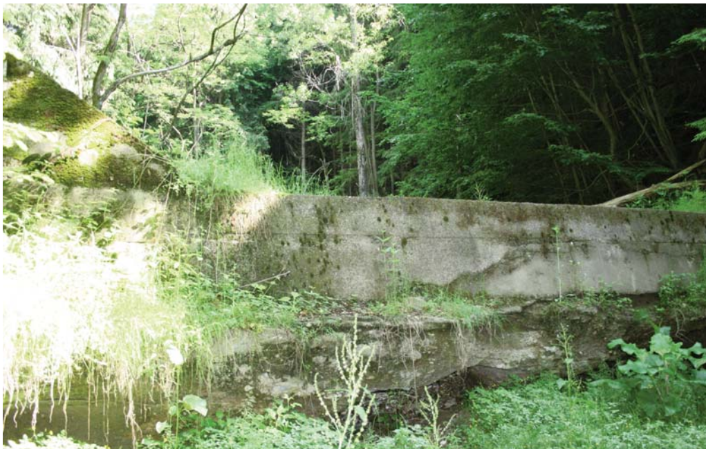
Fig. 6. 46 Pragul 16B1,0 de pe Valea lui Anghel, scos parțial din funcțiune prin evenimentul subminare (foto: Tudose 2009). The decrease in efficiency of sill no 16B1.0 on Valea lui Anghel after it had been affected by undermining (photo: Tudose 2009)
